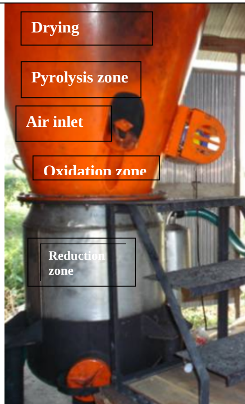
Figure 4: 9KW gasifier installed in CelAgrid, Cambodia (Source: T R Preston, unpublished data)
