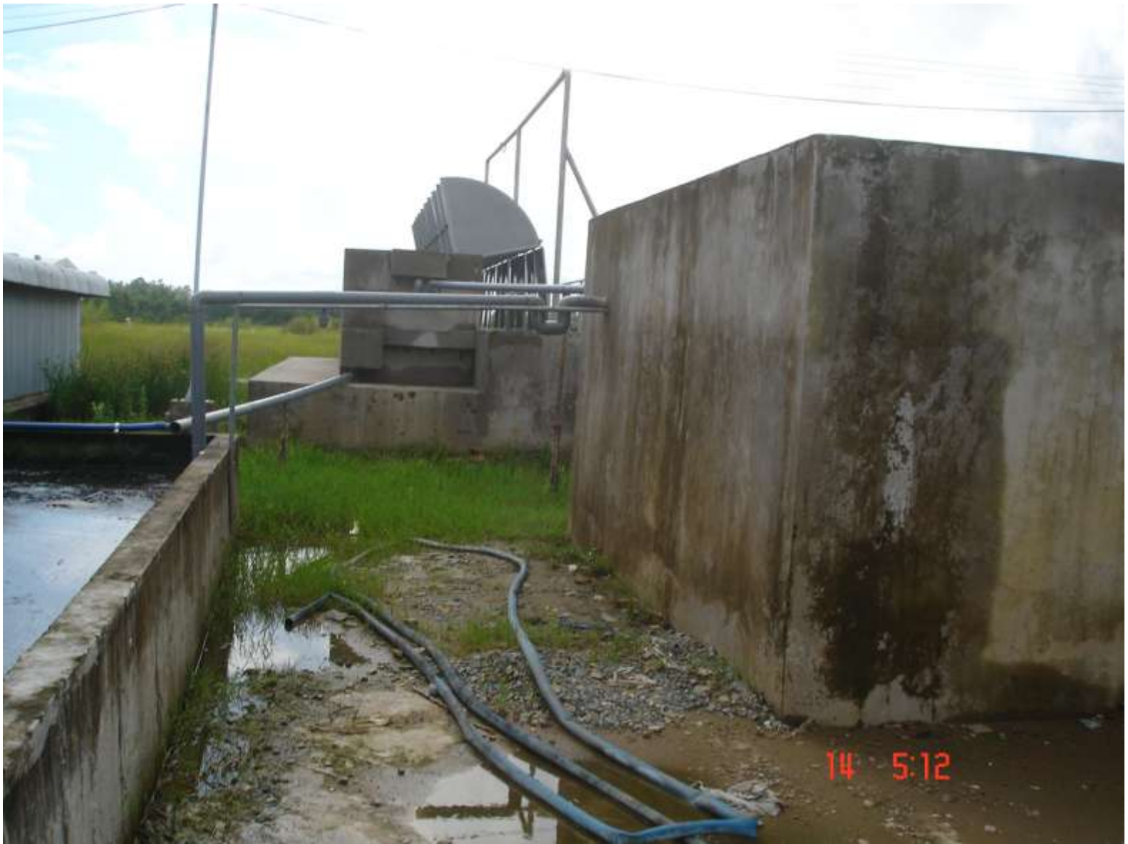
Biogas digester & hydrolyzed plant system
