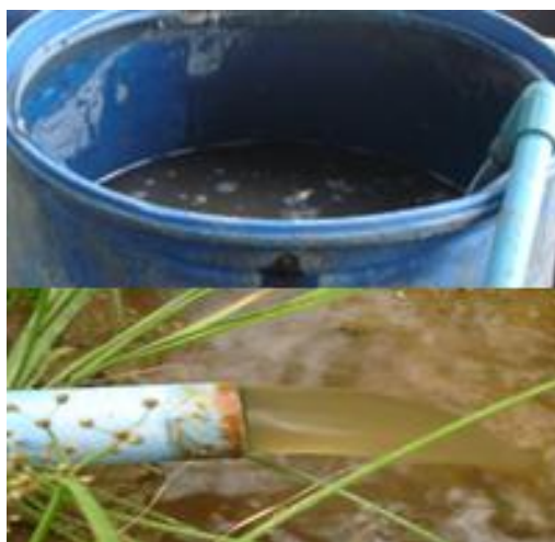
Photo 7: Effluent flow system to its treatment
