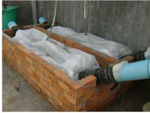
Photo 5: The plug-flow tubular polyethylene biodigesters
