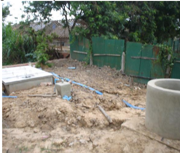
Photo 8: Concrete biodigester (high biogas pressure)
