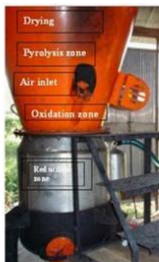
Photo 9: The 9 KW downdraft gasifier (Ankur Technologies) gasifier installed in CelAgrid, Cambodia
