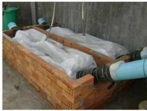
Photo 5: The plug-flow tubular polyethylene biodigester
