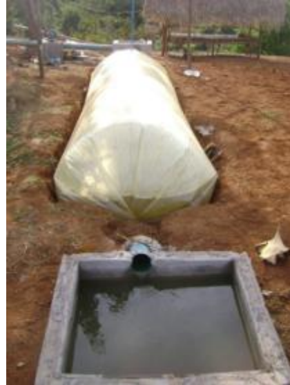
Photo 5: Effluent from the plug-flow tubular polyethylene biodigester
